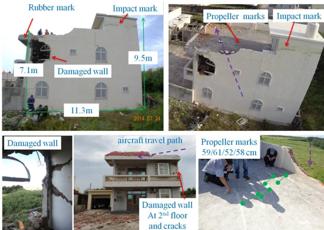
Figure 1.12-9 Initial aircraft impact, propeller, and rubber marks on building
