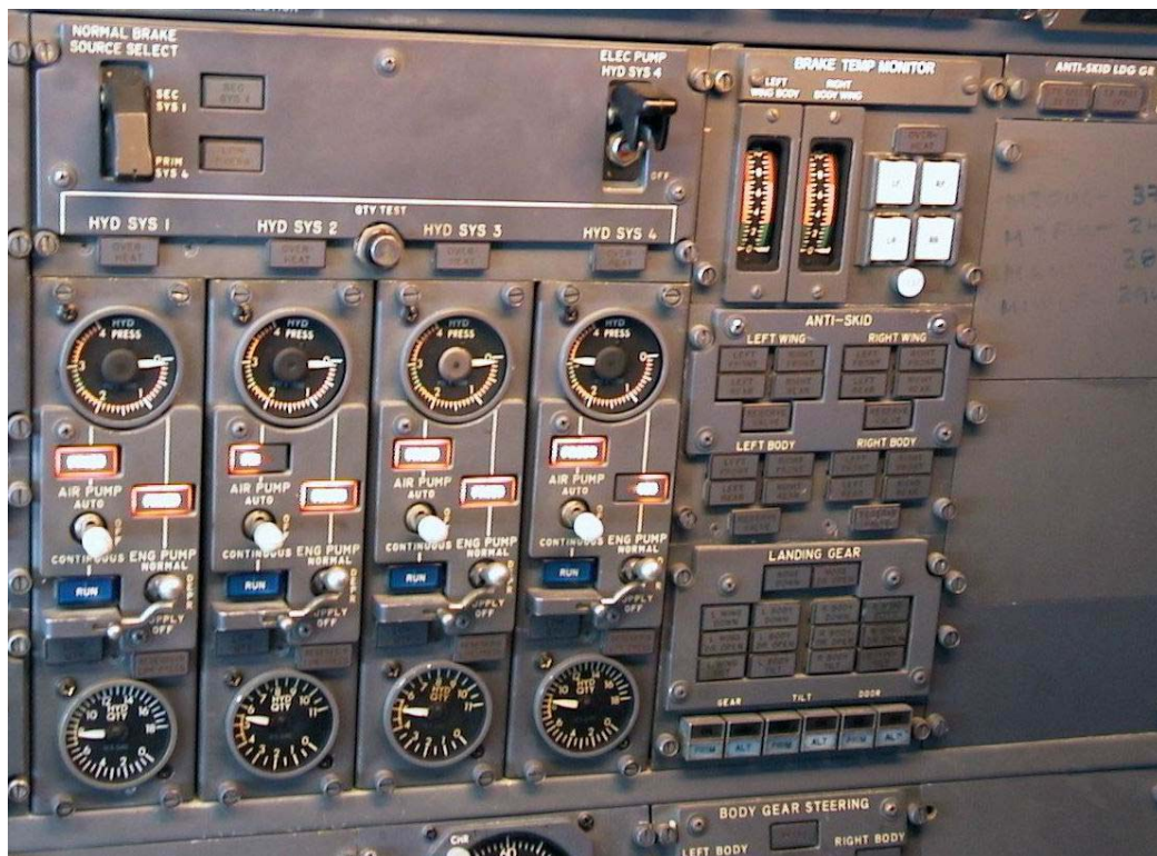
CM-3 Panel. ACP switch (labeled "ELEC PUMP HYD SYS 4", cover lifted) noted. Pressure gauge of Hyd. System No. 4 shows 3100 PSI.
