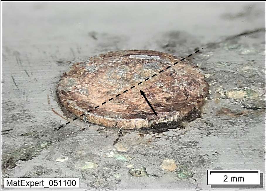
Figure 24: Severely corroded rivet N5. The black dashed line indicates the position of the microsection and the arrow indicates the direction the microsection surface was viewed from.
