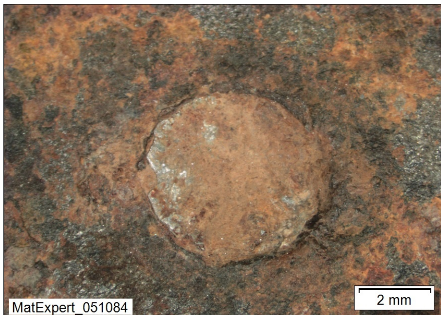
Figure 21: Close-up – broken rivet N4 with severe corrosion.
