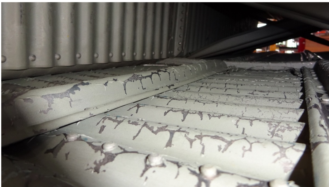
Figure 15: Inside of the horizontal stabiliser – areas where the anti-corrosion paint had partially flaked off.
