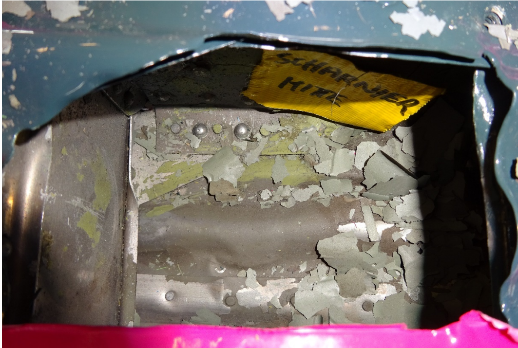
Figure 16: Flaked off anti-corrosion paint on the inside of the left elevator.
