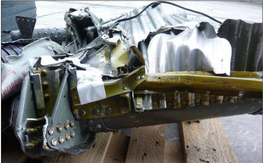
Figure 11: Repairs carried out in the centre wing, apparent by the greenish-yellow structural parts and the golden yellow connecting elements.
