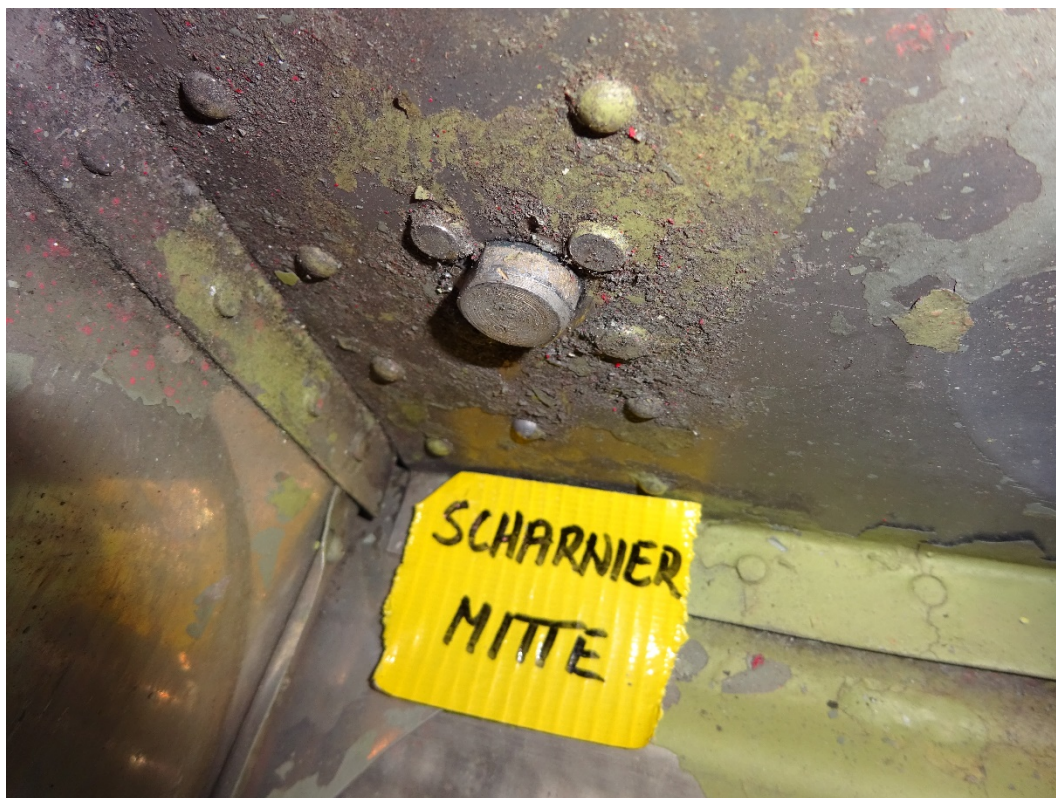
Figure 17: Inside of the rudder – head of the bolt for attaching the central hinge; lack of anti-corrosion paint; corrosion on sheet metal, rivets and bolt (label text reads central hinge).
