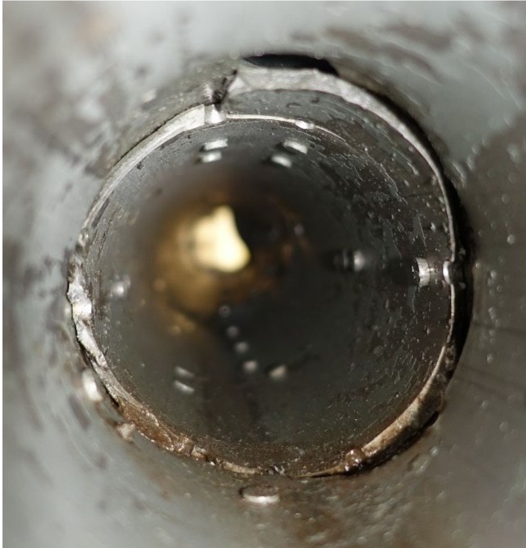
Figure 13: Close-up of the inside of the spar tube where fractures were found.
