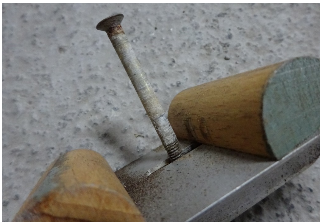
Figure 8: Severely corroded bolt for mounting a seat rail.
