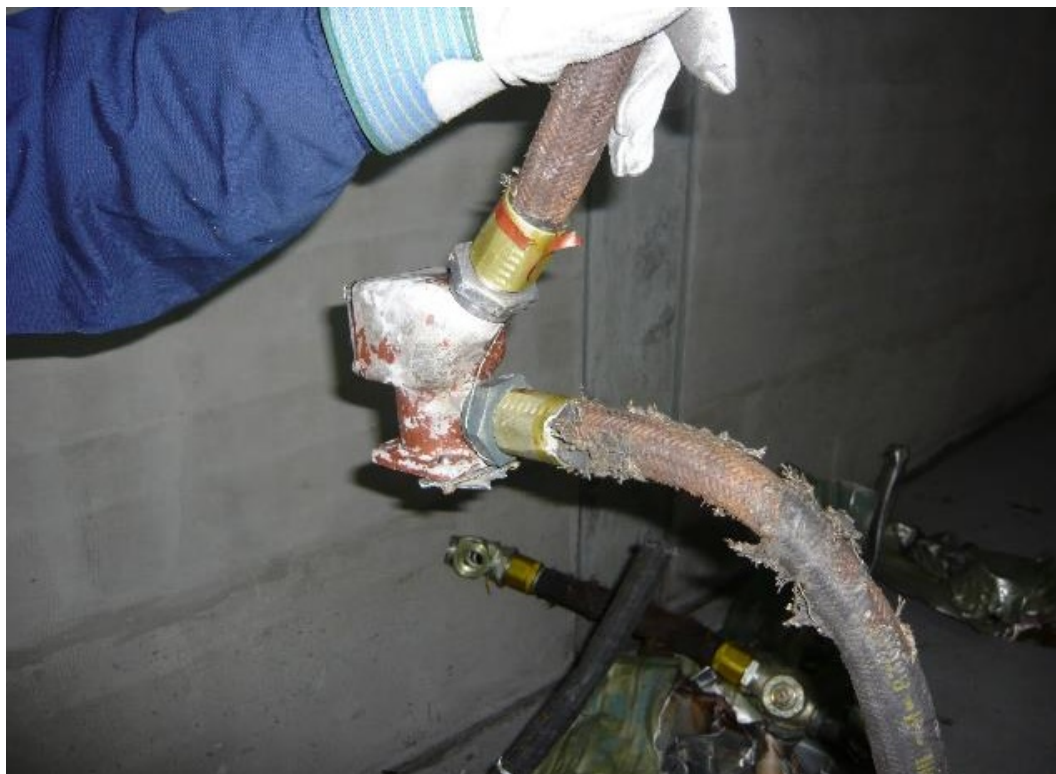
Figure 30: Lines show obvious signs of decay due to age.
