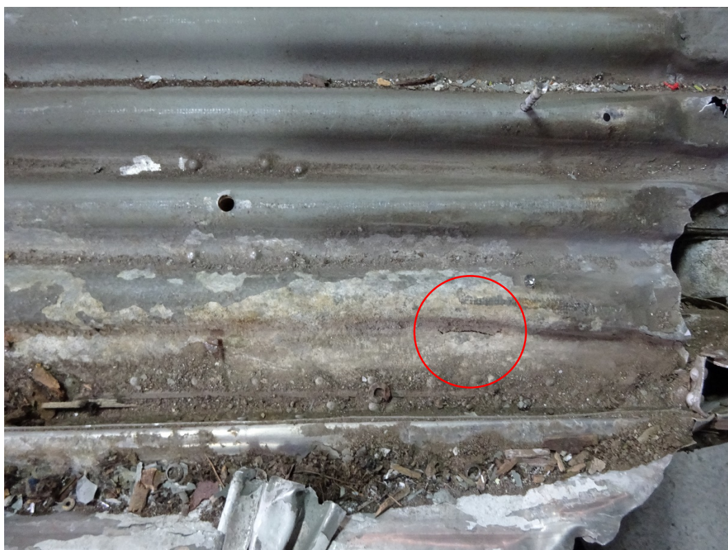
Figure 6: Close-up of figure 2 number (4) – severely corroded floor structure with fracture (red circle).
