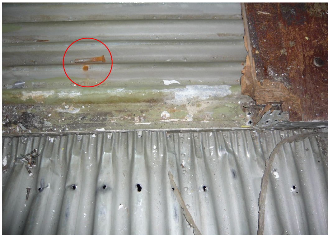
Figure 4: Close-up of figure 2 number (2) – severely corroded floor structure and bolts (red circle).
